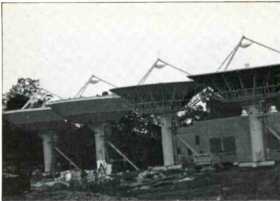
The new HBO ground communications station at Hauppauge, New York under construction last summer. (Photo by Tony Earll, KNY2AE)
